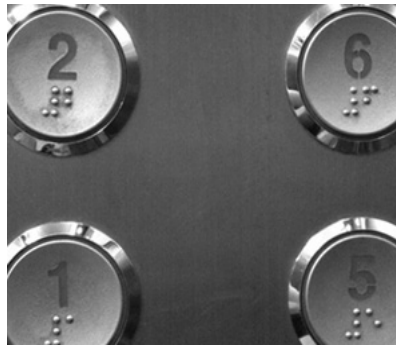
Figure 14 Button of elevator
